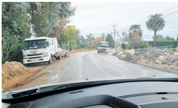
Evidence of Cyclone Gabrielle's damage is evident on the way to Waiohiki.
